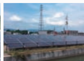
Wakayama Solar Power Plant
