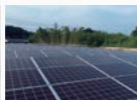
Kagoshima Solar Power Plant
